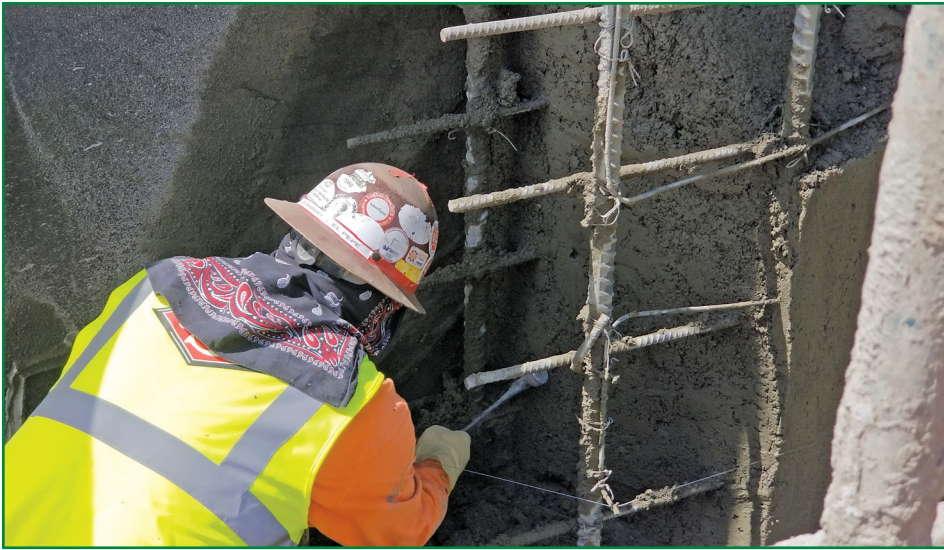
Figure 3 – During placement of shotcrete, installation of an additional striker pin was observed, which created penetrations in the waterproofing membrane that could not be detailed by the waterproofing installer.
