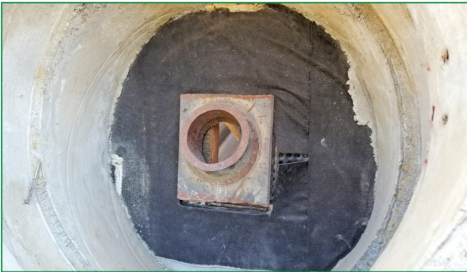
Figure 7 – Earth retention tie-back observed after form work was removed prior to the application of waterproofing detailing.
