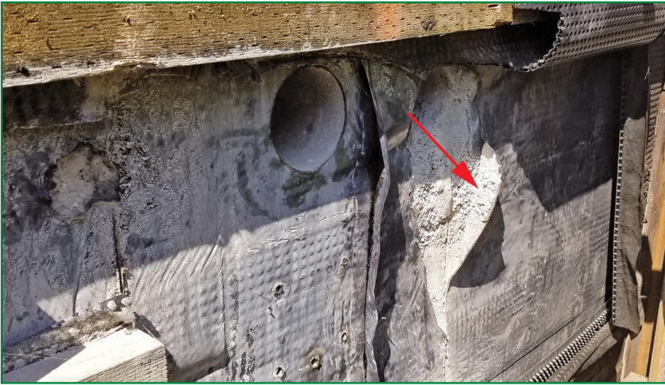
Figure 5 – Observations from the backside of the mock-up showed the membrane did not bond in the oversprayed shotcrete areas (see arrow).
