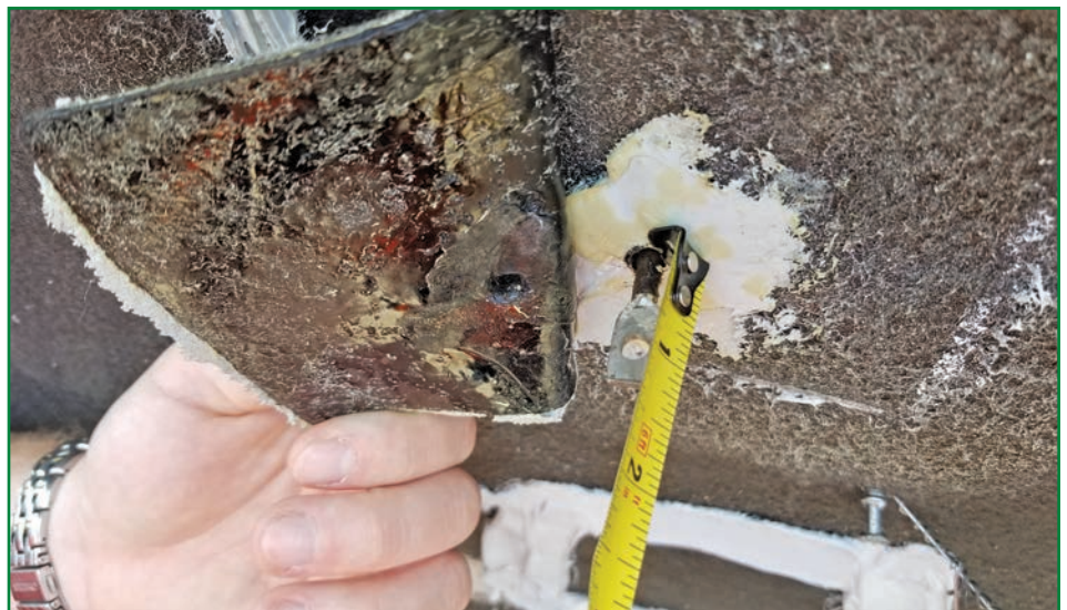
Figure 4 – Striker pin installed and detailed with waterproofing was observed to be inadequate, demonstrating a difficult detail to achieve repeatedly in the field.
